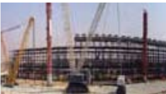
ASAB Gas Development Phase II Abu Dhabi, UAE
