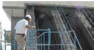
Sewage and Drainage Pumping Station Abu Dhabi, UAE
