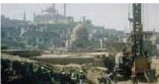
Sanitary Drainage Cairo, Egypt
