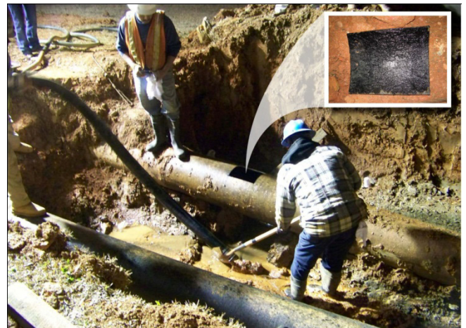
A force main coupon is used to assess this damaged pipe's integrity and the extent of necessary repairs
