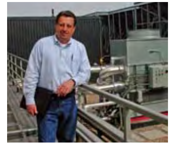
Steve Mancuso Facilities Maintenance Manager for the CH2M HILL Headquarters Campus
